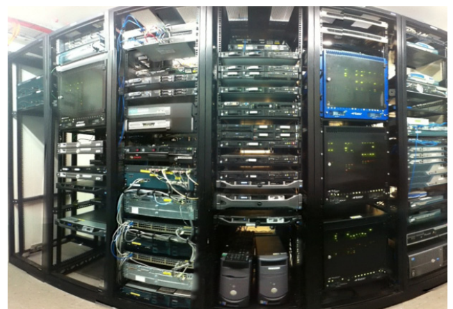
ASC's Adelaide Equipment Room
